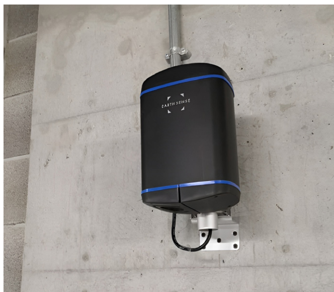
Figure 6: Mains powered Zephyr® deployed on a concrete wall in one of the underground areas at Expo 2020 Dubai.
